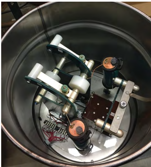
Figure 49: A 20-gallon oil drum contains the three Ross HV relays used in the charging circuit. The relays are operated by the control panel during the charging sequence. The large copper-sulfate dump resistors in this photograph were ultimately replaced with 50-k \Omega ceramic resistors to minimize maintenance.
