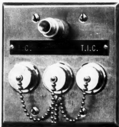
Figure 1--One of the 68 junction boxes in the distribution system at NNMC. Top junction is for TV and program audio, originating or receiving; left, for conference intercommunication; right, system intercommunication; center, spare.
