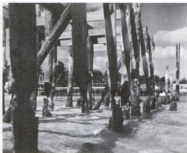
Marine organisms were responsible for much of the damage to these pilings. (Photo by R.D. Reid, ONR)
