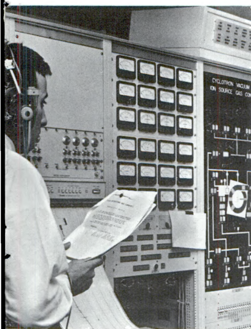
Above: Artist's concept of NRL's new cyclotron facility. Left: Part of the control panels for the cyclotron and beam transport system. Lower left: The 250-ton magnet where particles are accelerated (right) and the resonator tank. The two units will be joined together when finished. Lower right: Experimental room #3, looking towards the beam slot. Some of the concrete blocks will be replaced by a steel shutter to allow the beam to enter. The cyclotron and beam preparation equipment are on the other side of the 9-foot thick wall.
