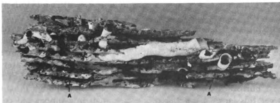
Figure 5 — A fragment of wood damaged by teredinids and limnoria. The white tubes are the calcareous burrow linings produced by the teredinids. The softer spring-wood was rasped by the limnoria (A).
