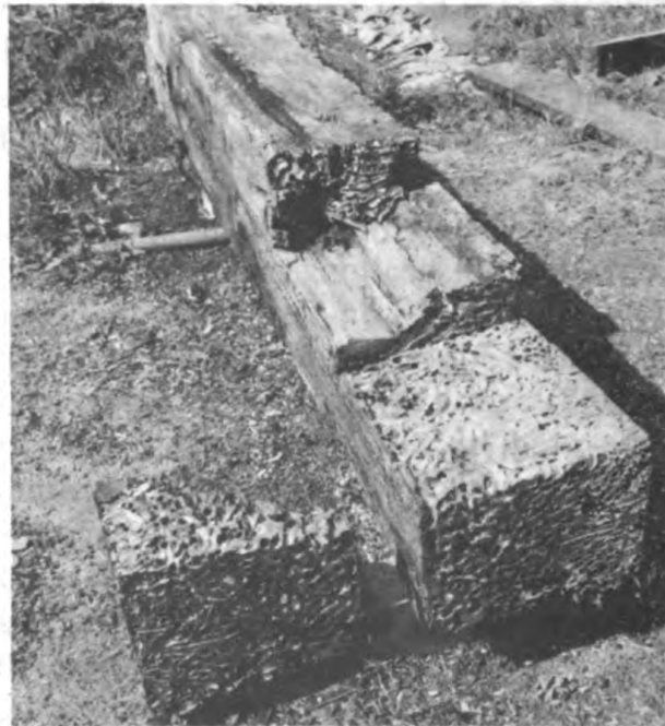
Figure 1 — Fender timber thoroughly infested by teredine borers. The outer surface of the wood gives the untrained observer little indication of the extent of internal damage that has occurred.
