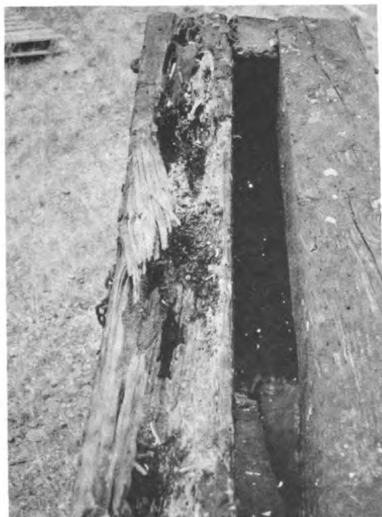
Figure 8 — Section of a camel (used between ship hull and pier) showing extensive damage to a lower member caused by the combined action of teredinids, pholads, and limnoria.
