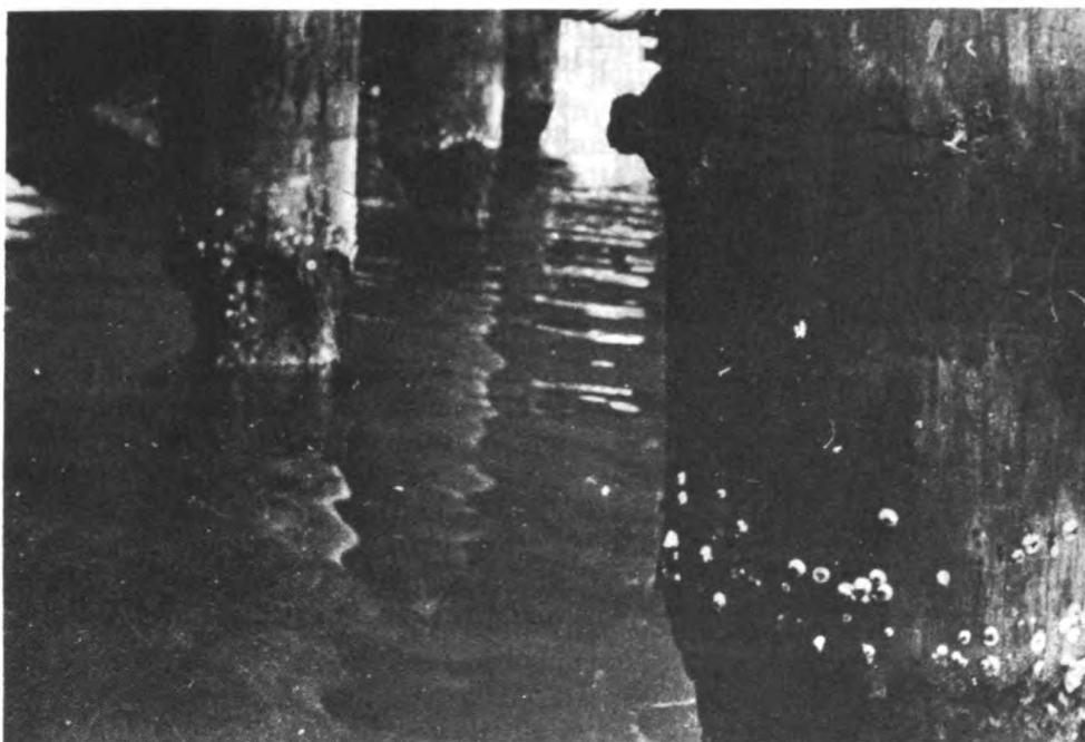
Figure 5. These piles, supporting the Fort Sherman Dock, show the work of the water flea.
