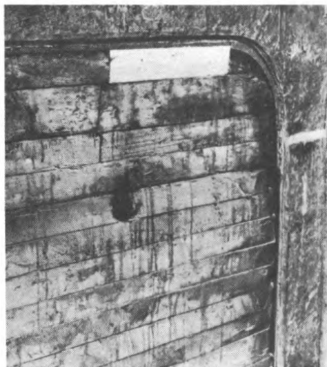
Balsa wood-filled blister void
