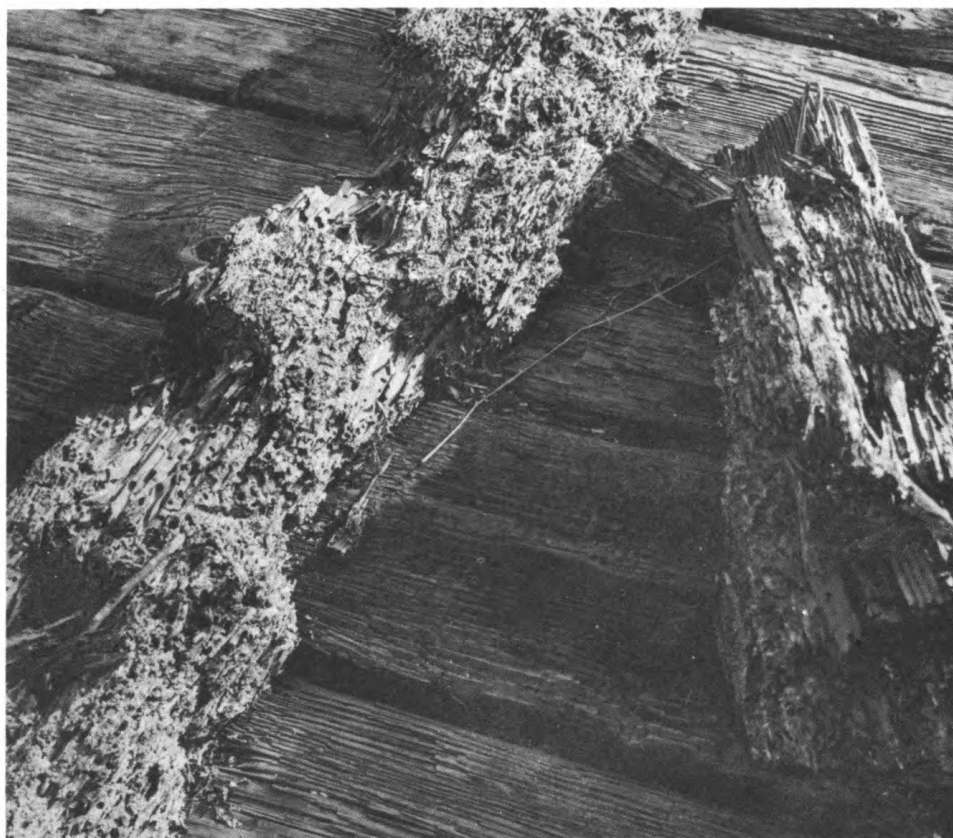
Figure 1 - Destruction of marine timbers at a seaplane ramp location, Guantanamo Bay, Cuba (1949). These timbers had been creosoted before being used in building the ramp, but in 15 months were reduced to a hopelessly weakened condition by vigorous attack from LIMNORIA and TEREDO. The long channel-like borings of TEREDO are frequently uncovered (as shown above) by the borings of LIMNORIA which characteristically work inward from the surface. The combined activity of borers such as these compound the deterioration and hasten the failure of marine timbers.
