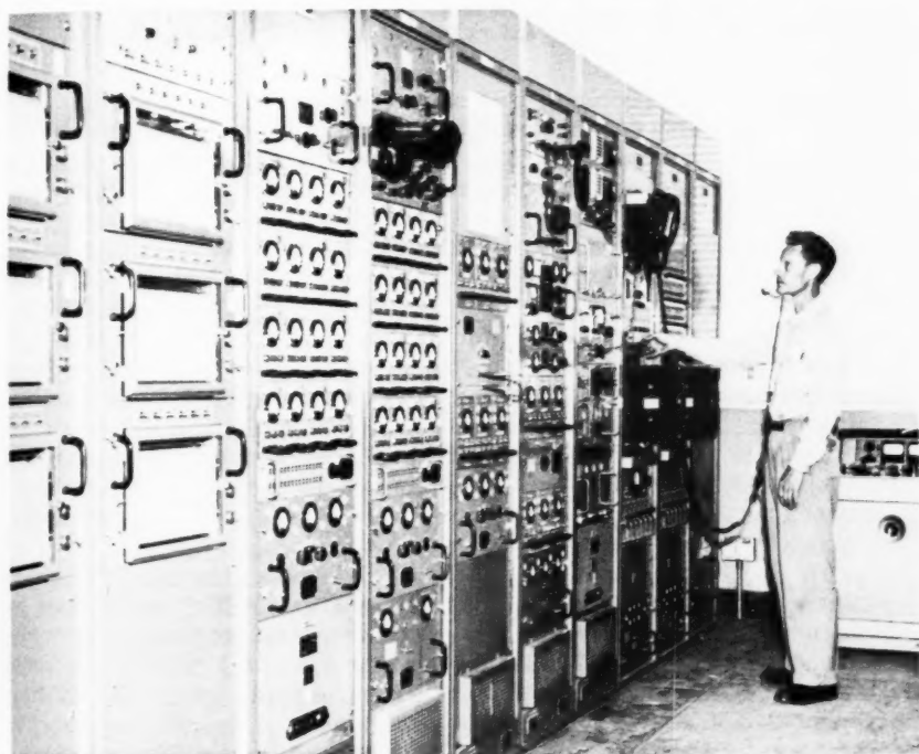
Figure 4 - UNR-5 telemetering receiver.
